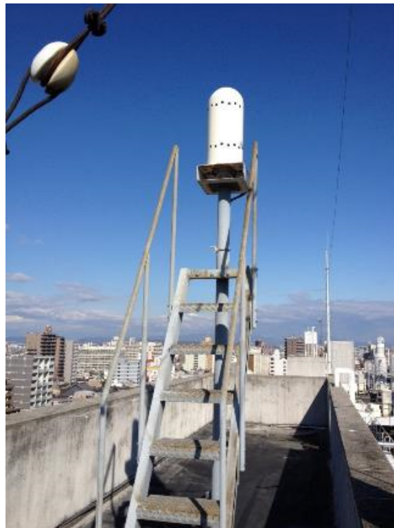
Figure 5.4 Example of installation at a height of dozens of meters above the ground (Aichi Prefecture)
