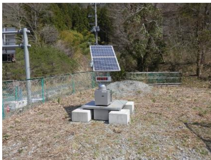
Figure 5.6 Example of the installation status of a transportable monitoring post (the positioning of the detector: 1 m above the ground, with solar power generation and external battery facilities)
