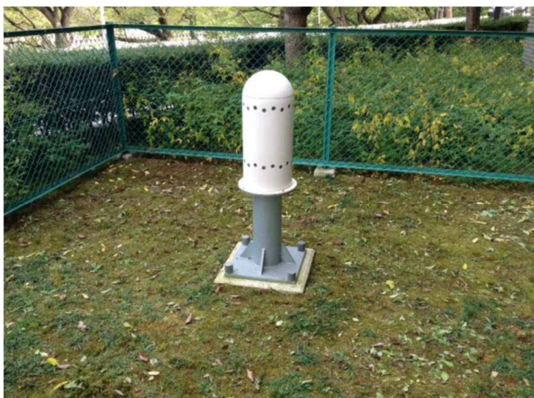
Figure 5.1 Example of installation on an alley, at a height of 1 m above the ground (Aichi Prefecture)
